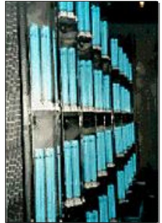
UVGI lamp array installed inside the air handling units
